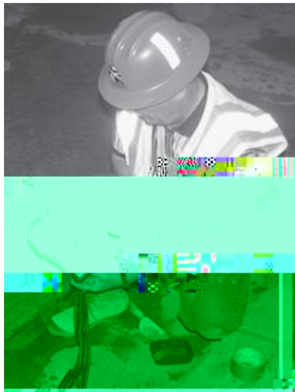
Figure 6: Concrete maturity monitor
